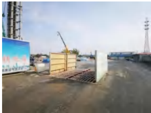
(46)南通火车站洗车槽 2021.11
