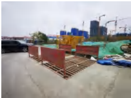
(117)园林路站洗车槽 2021.11
