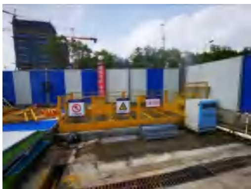
(139)通富路站三级沉淀池 2020.7
